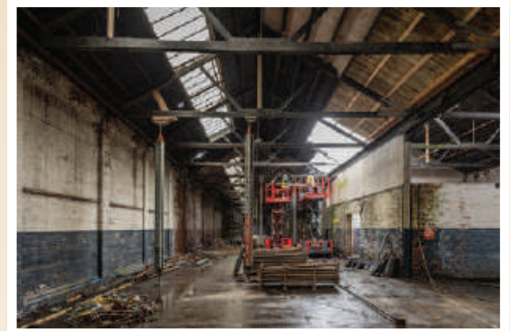
Dundee Tram Depot, ready for a new life Credit: Dundee Museum of Transport
